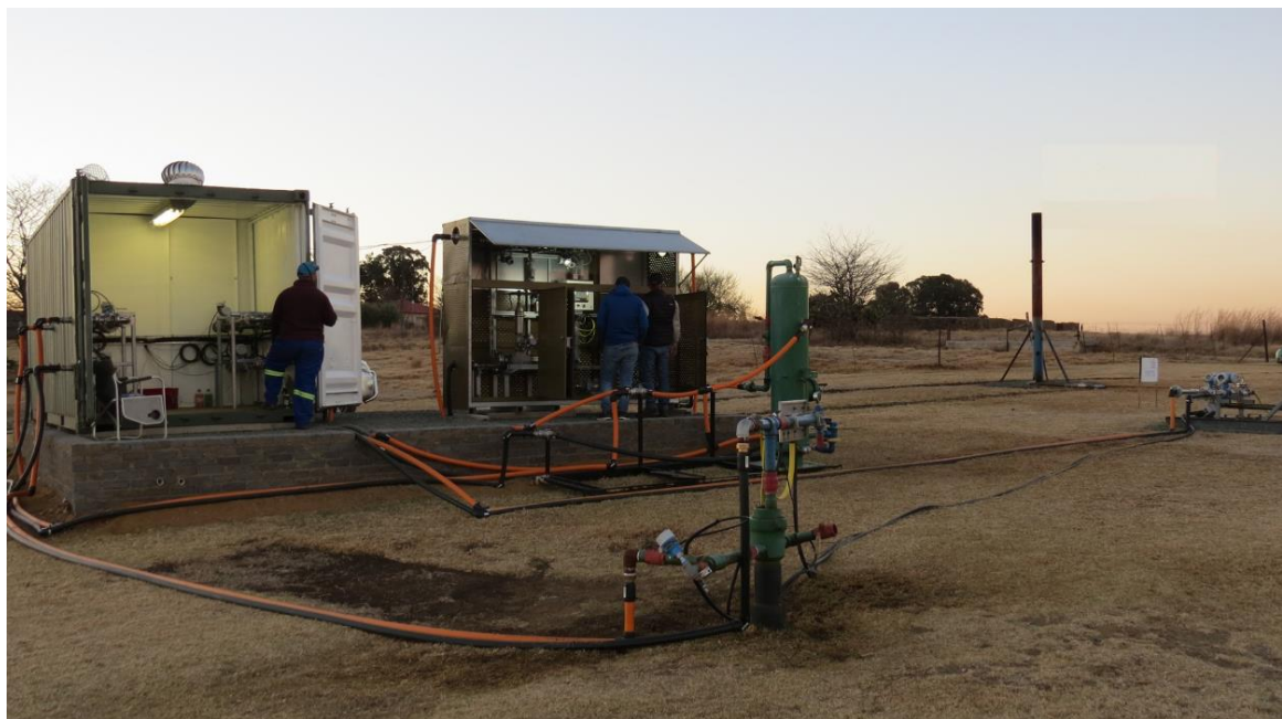
Figure 2. – Gas separator and well head equipment on Well KA-03PTR
