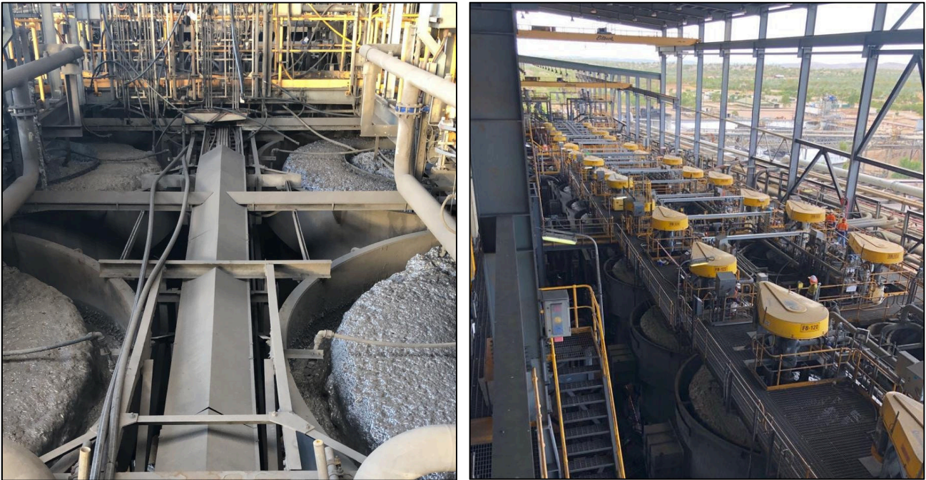
Figures 3 & 4: Cleaner 1A operational and 1B now online (left) & installation of pipe racks as part of the refurbishment and upgrade of launder spray and reagent dosing systems (right)
