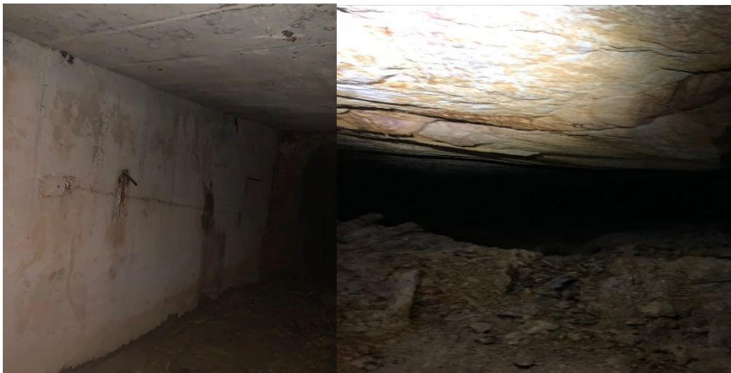
Image 5: Good condition reported of the Qala Adit shaft infrastructure (left) and the K9A hanging wall (right)
