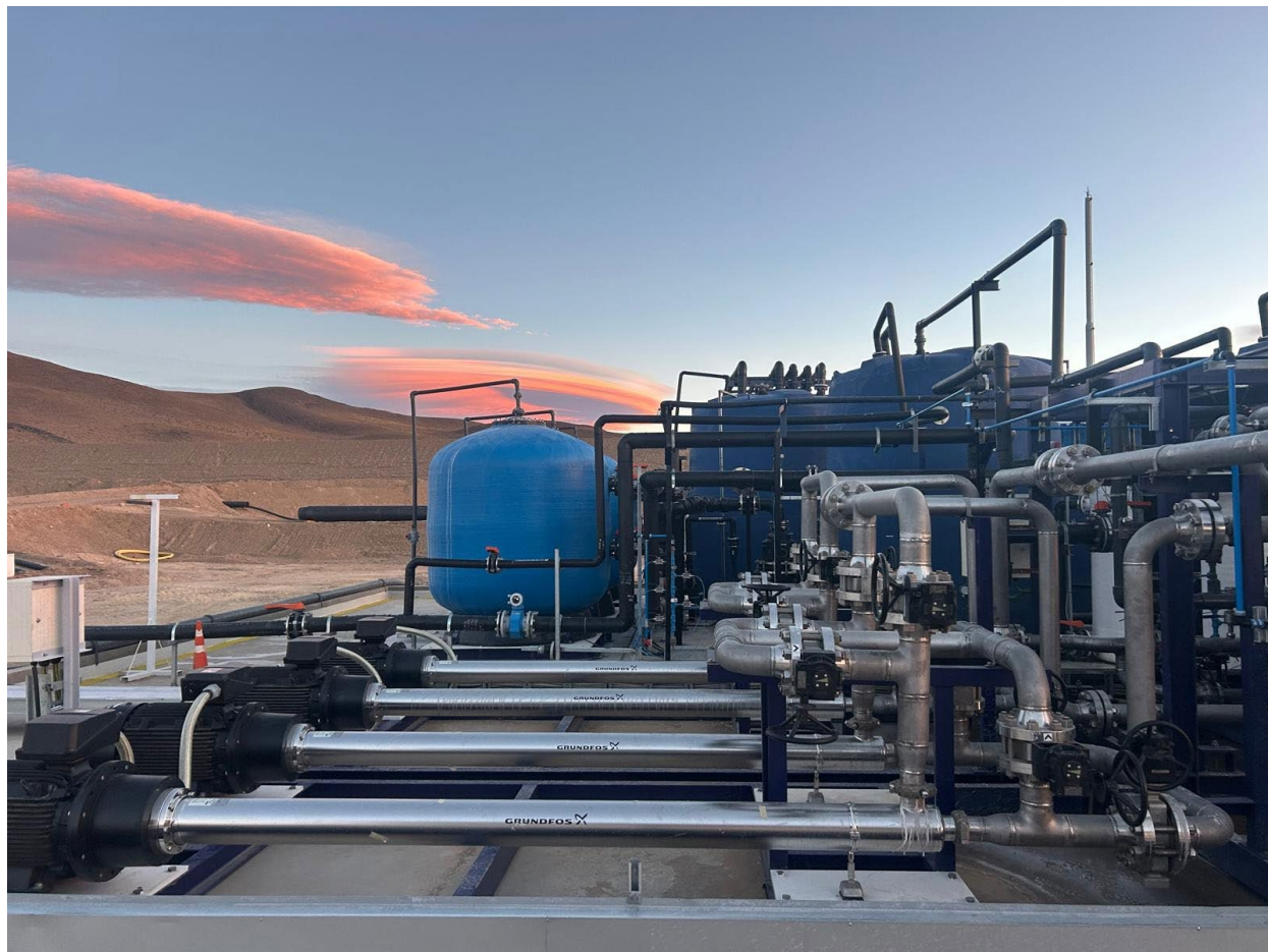
Figure 2. HMW nanofiltration plant in operation.
