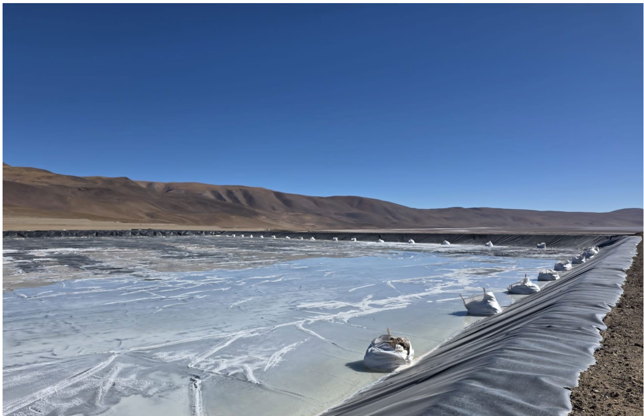
Figure 1. Processed brine discharged into final evaporation pond.
