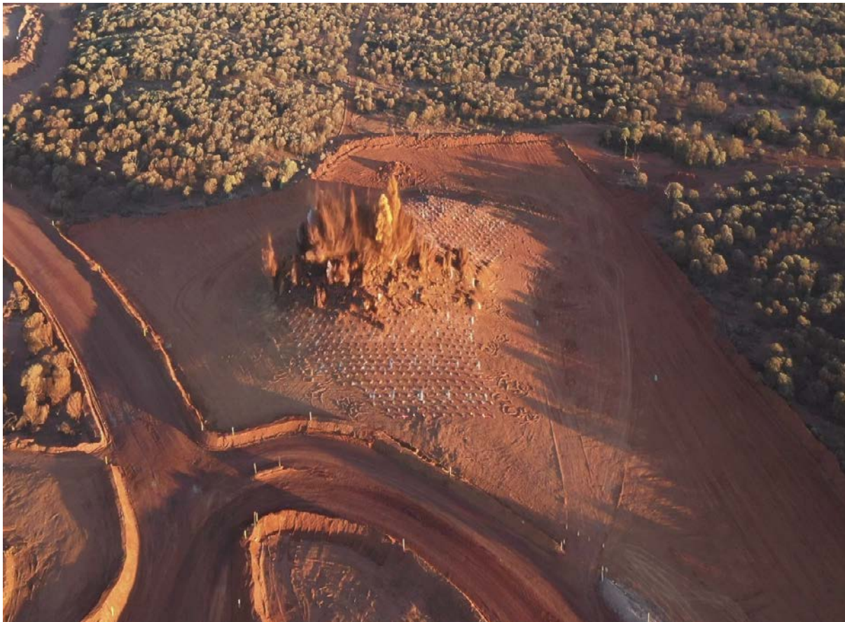
Figure 1: : C4 Stage 2 – First Blast that occurred on 22 nd June 2021 at the South End of the Stage 2 Pit
