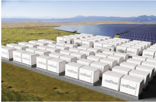
Breakthrough Multi-MWh project in US
