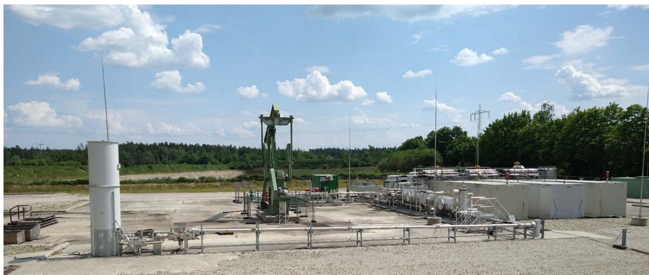
Figure A3: Image of the leased production unit which will be used at the Anshof field and drilling location.
