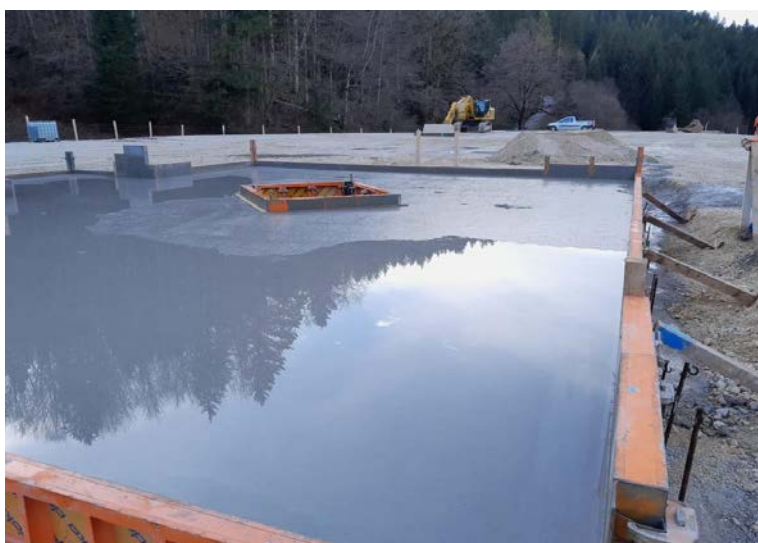
Well site construction at the Welchau-1 drilling location in the Northern Calcareous Alps
