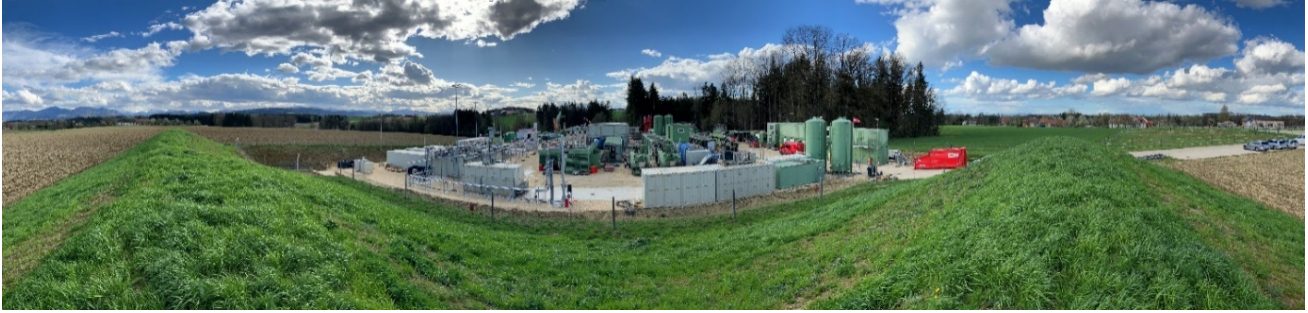
Figure 2: Anshof Permanent Production Facility at ADX' Anshof-3 location
