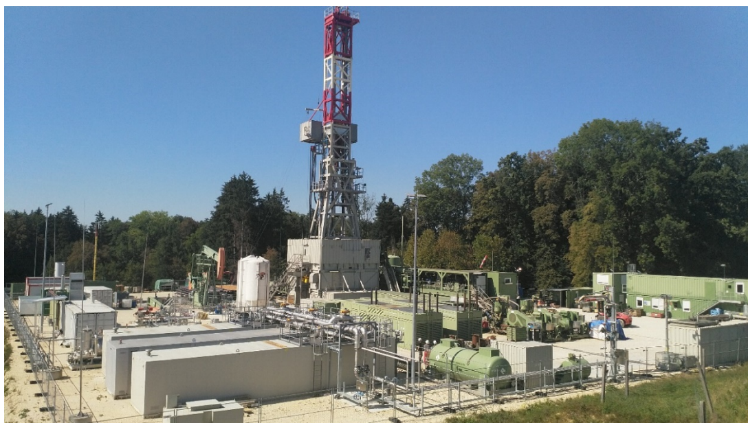
Figure showing the RED E202 rig drilling the ANS-2A well at the Anshof PPF location. On the left hand side of the rig the rod pump on the Anshof-3 discovery well can be seen.
