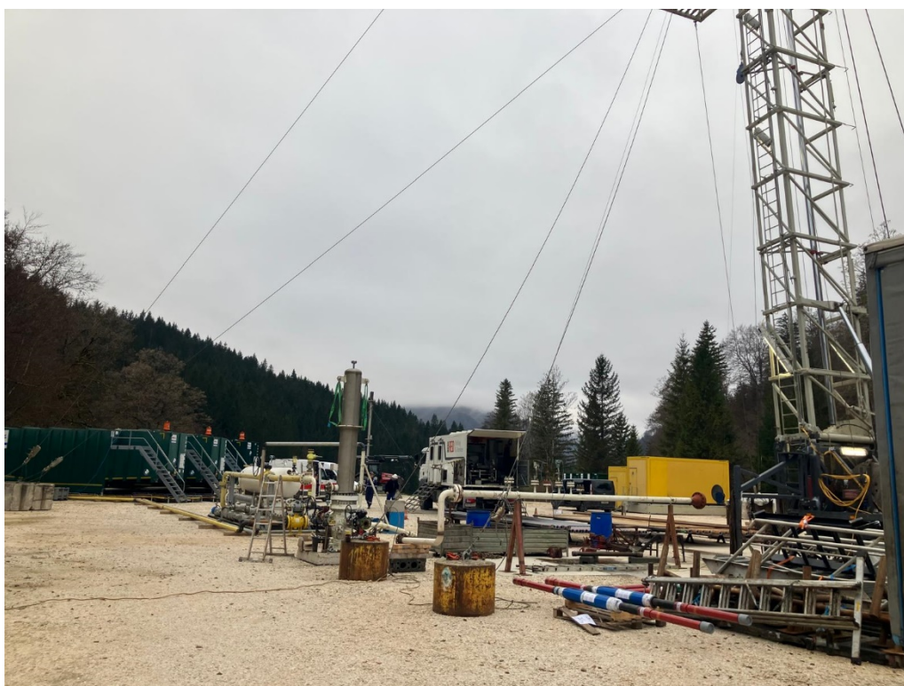
Well completion work and Flow Testing Facilities set up at the Welchau-1 well location for flow testing the well
