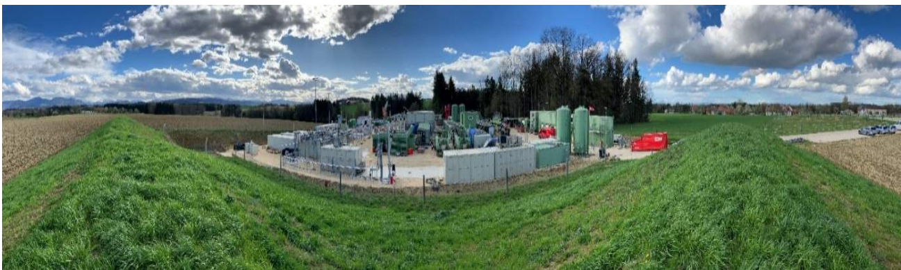
Figure 3: Anshof Permanent Production Facility at the Anshof-3 location
