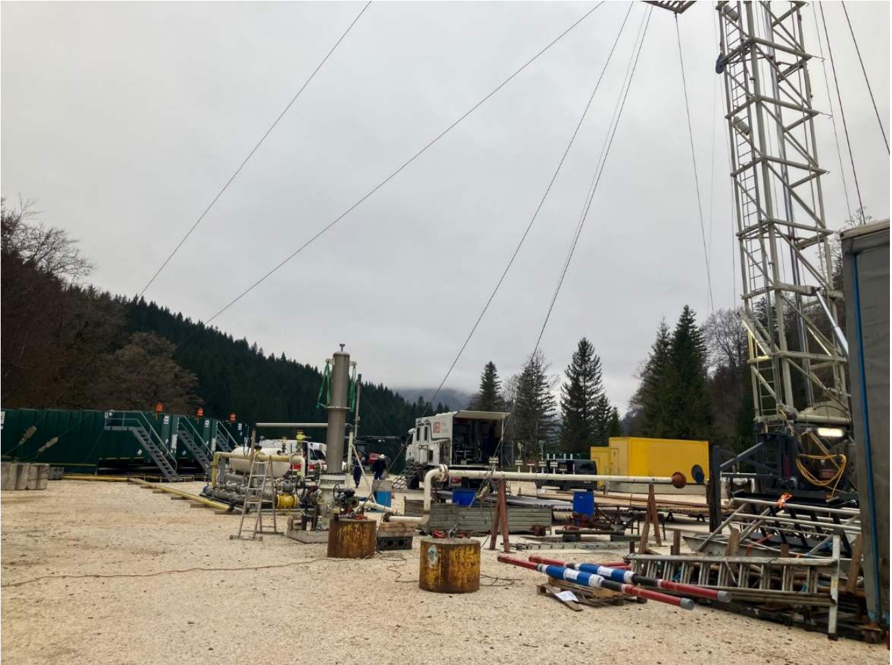
Figure 10: Well completion work and Flow Testing Facilities set up at the Welchau-1 well location
