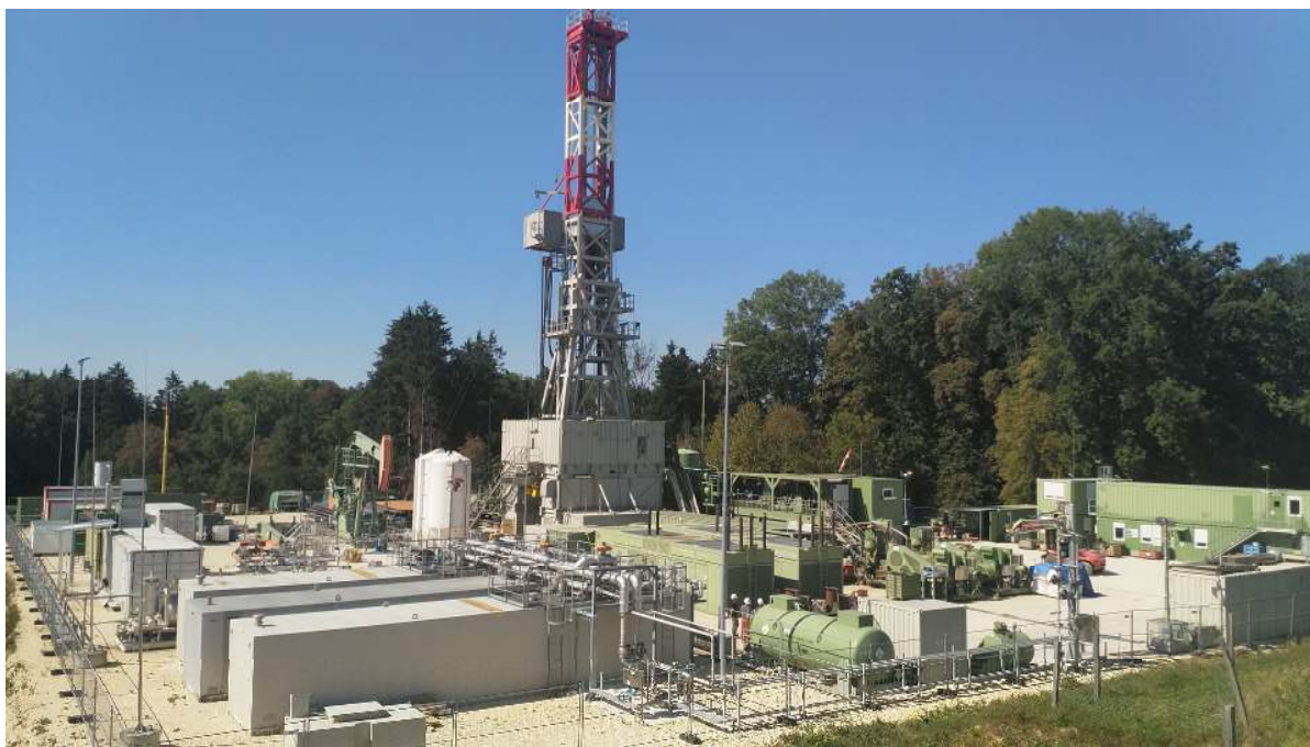
Figure 1: Drilling of Anshof-2A appraisal well and production operations at the Anshof Field in Upper Austria
