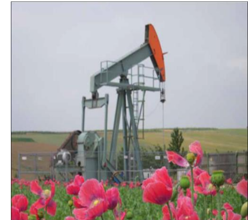
Zistersdorf & Gaiselberg Production Assets Vienna Basin, Austria
