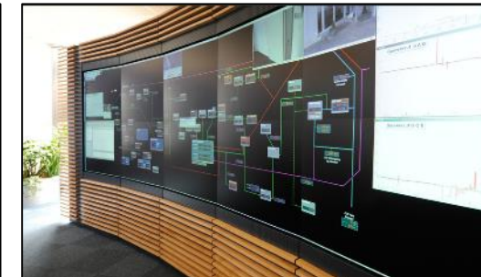
Central fully automatic dispatching centre
