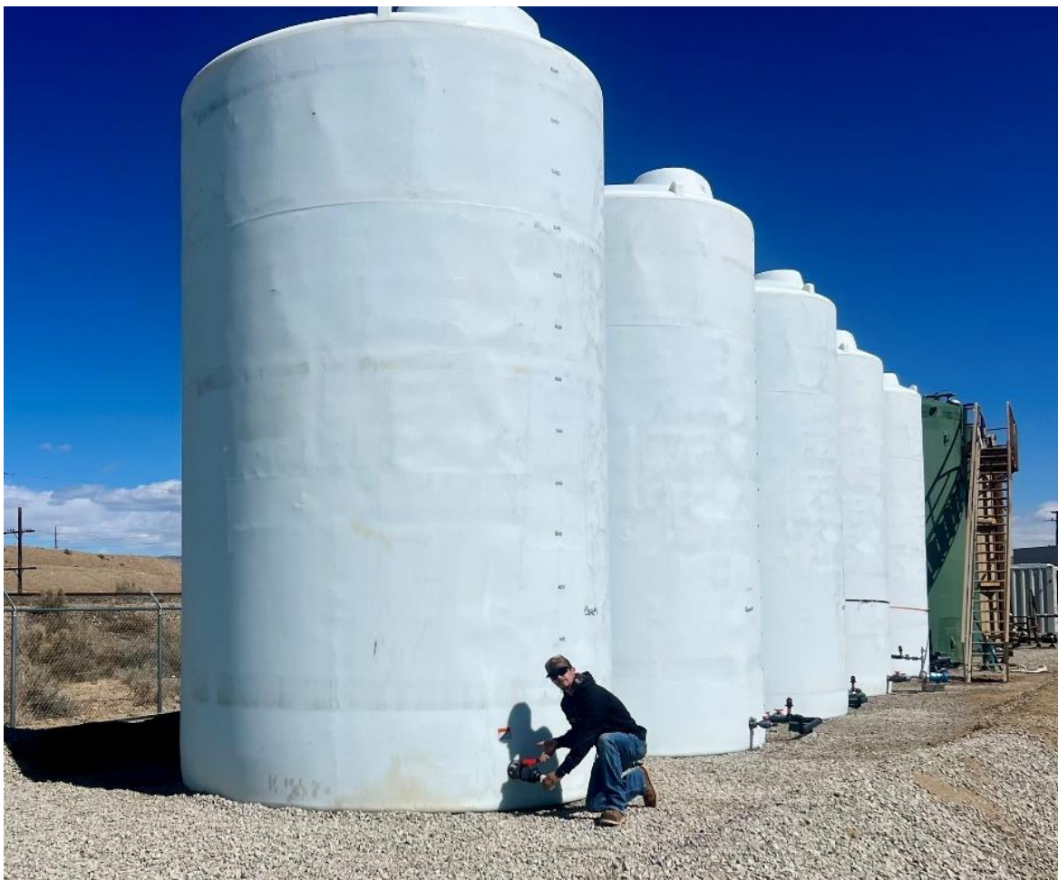
Figure 1: Photo showing the collection and sampling from the near full tanks of lithium chloride eluate produced using KTS DLE at Green River.
