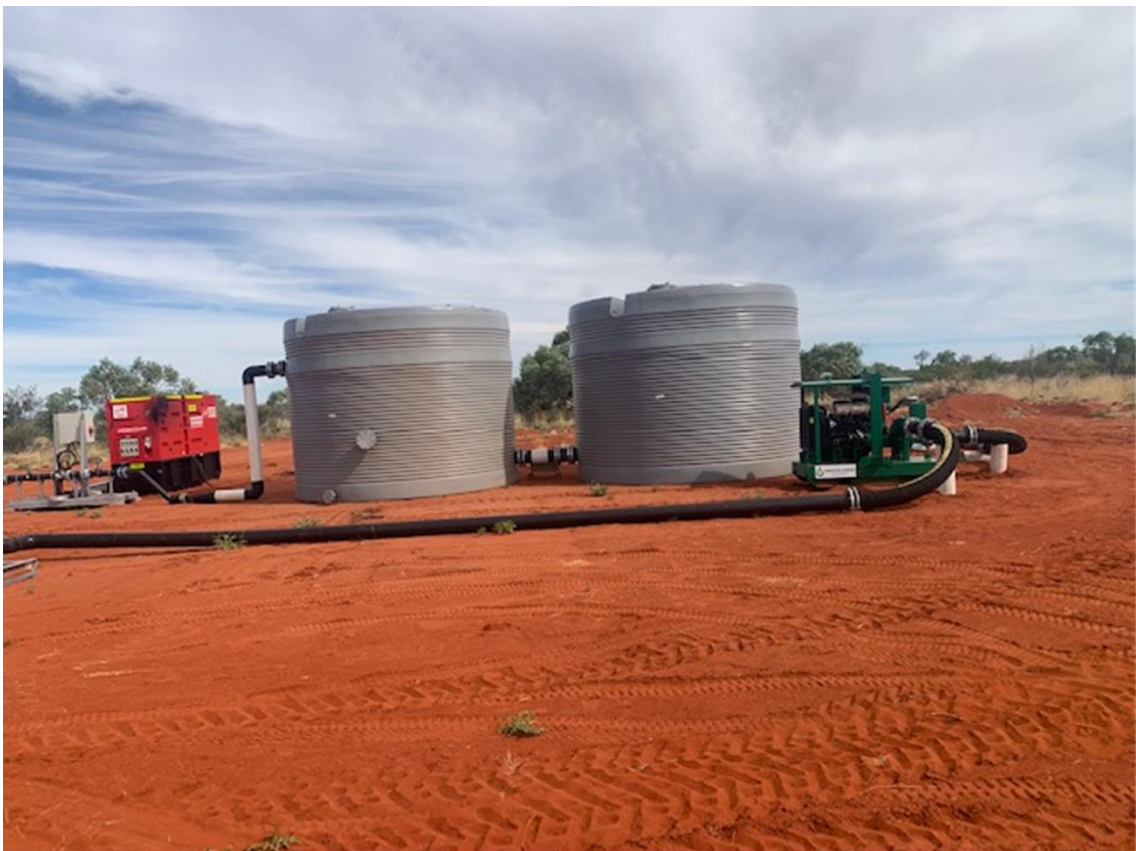
Figure 11: Borefield D temporary construction water supply tanks and pumps
