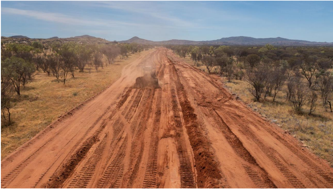
Figure 12: Clearing of the pipeline corridor between the Nolans borefield and the process plant site.
