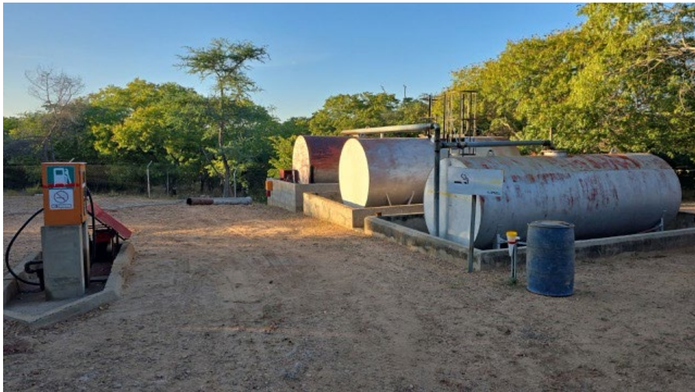
Figure 4: Diesel fuel storage tanks at Muntanga camp (57,000 litre capacity)
