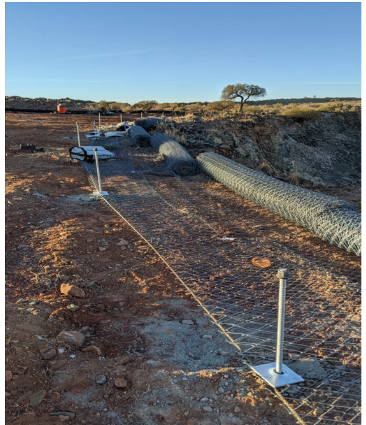
Ground support being anchored above the portal in preparation for securing to the Paris Pit wall face above and around the new portal.
