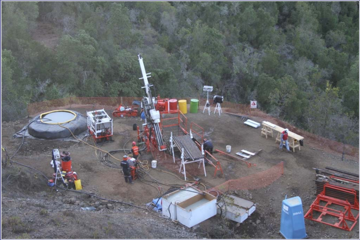
The new, purpose-built Assad rig set-up on hole 1 (YB-001-D) at the Yerba Project
