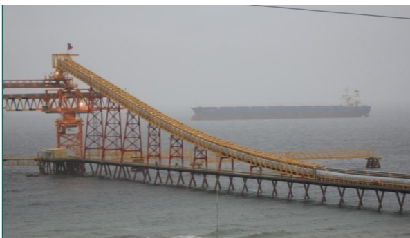
Photo 1. Coal loader at the recently commissioned 5mtpa Mina Invierno Chile's only large coal mine
