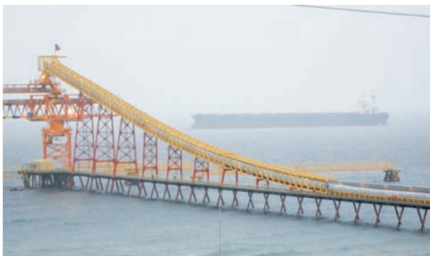
Photo 1. Coal loader at the recently commissioned 5mtpa Mina Invierno Chile's only large coal mine
