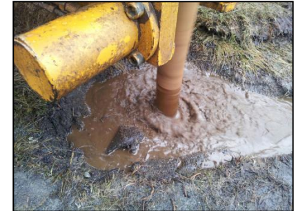
Brown drill water indicative of coal being drilled
