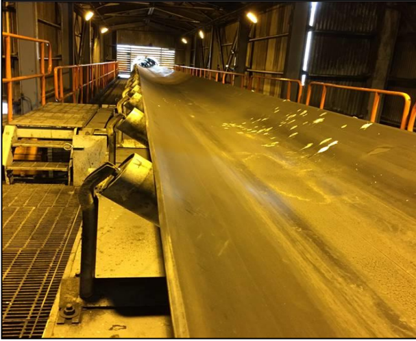
Photo 1. Conveyor System at Port Pecket
