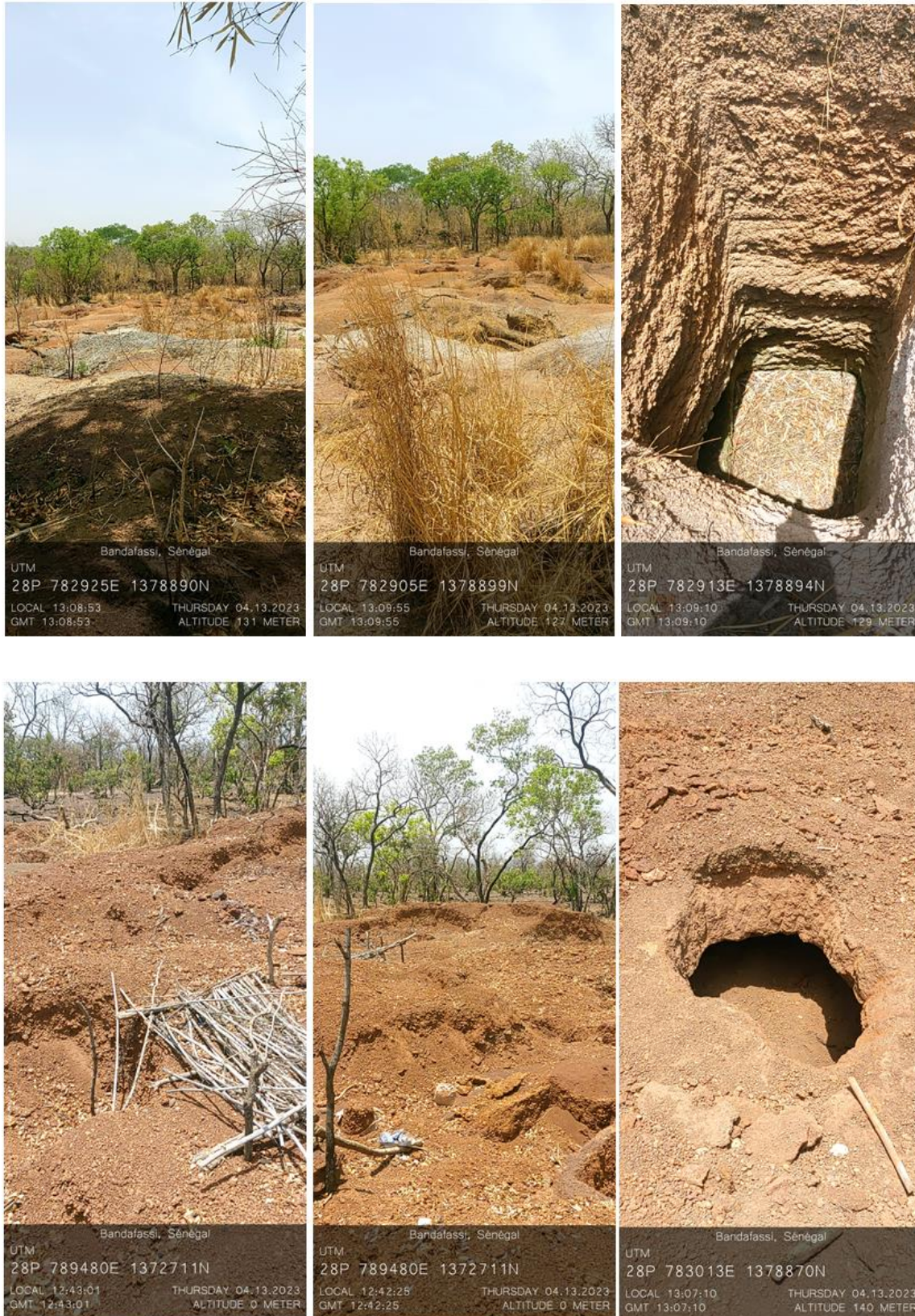
Figure 6: Photographs of artisanal gold workings in the Ibel permit area. Pits are up to five meters deep and reach saprolite. Mining is limited to the wet season when water for processing is available.
