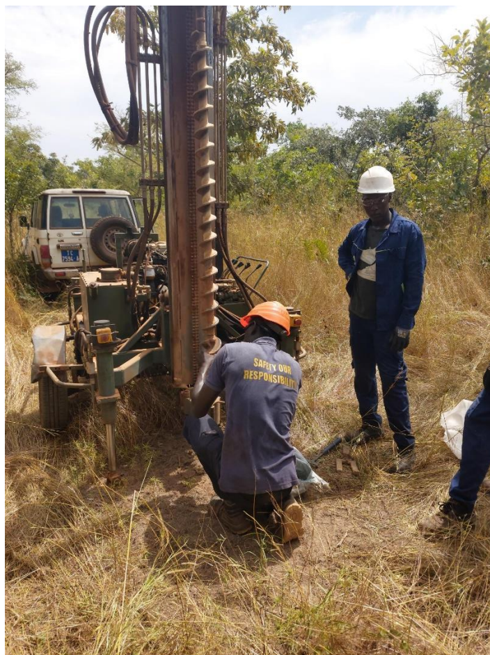
Figure 1: Testing the auger for penetration of laterite and depth potential – Saraya deposit
