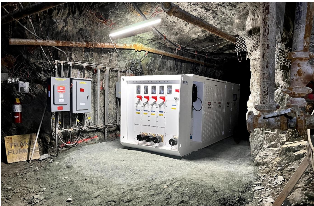
Figure 8: New underground Mine Power Centre installed at XC7.
