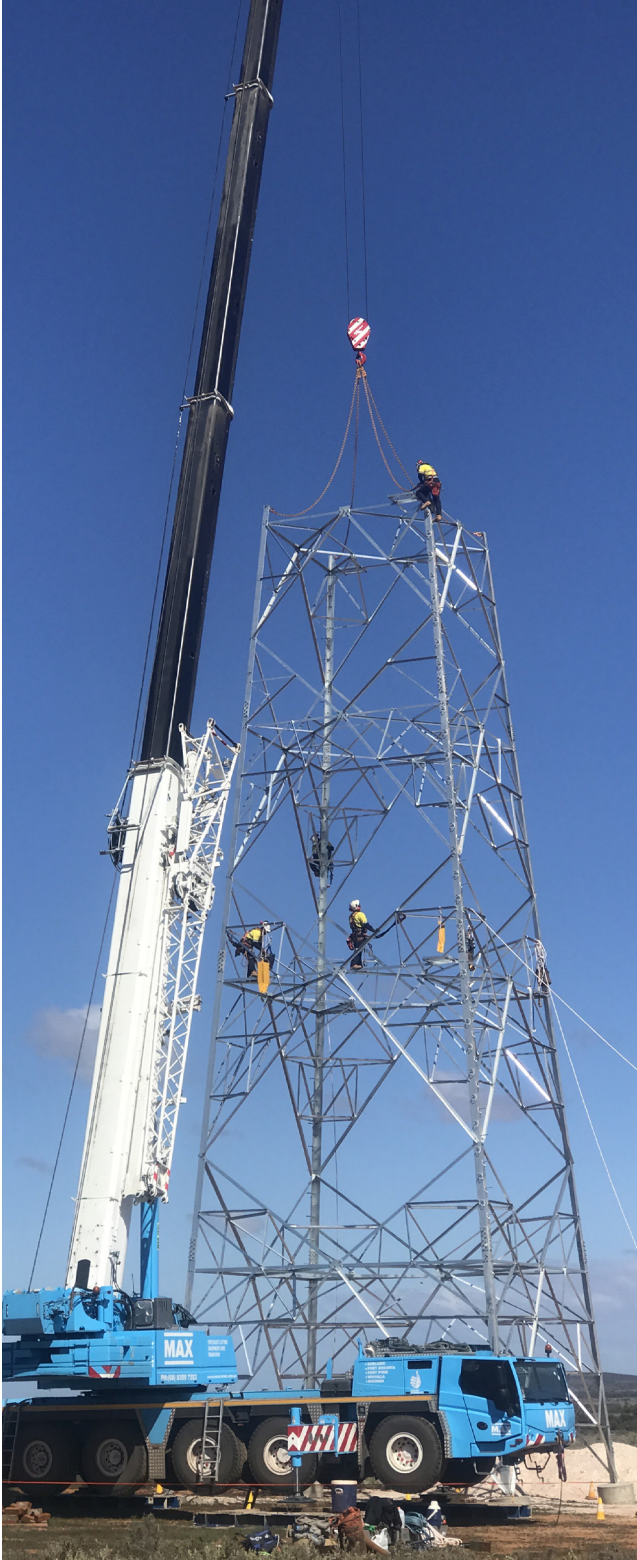
The Eyre Peninsula Link comprises a new 270 kilometre, high-voltage transmission line to be constructed from Cultana to Port Lincoln, via Yadharië (Image- Electranet)
