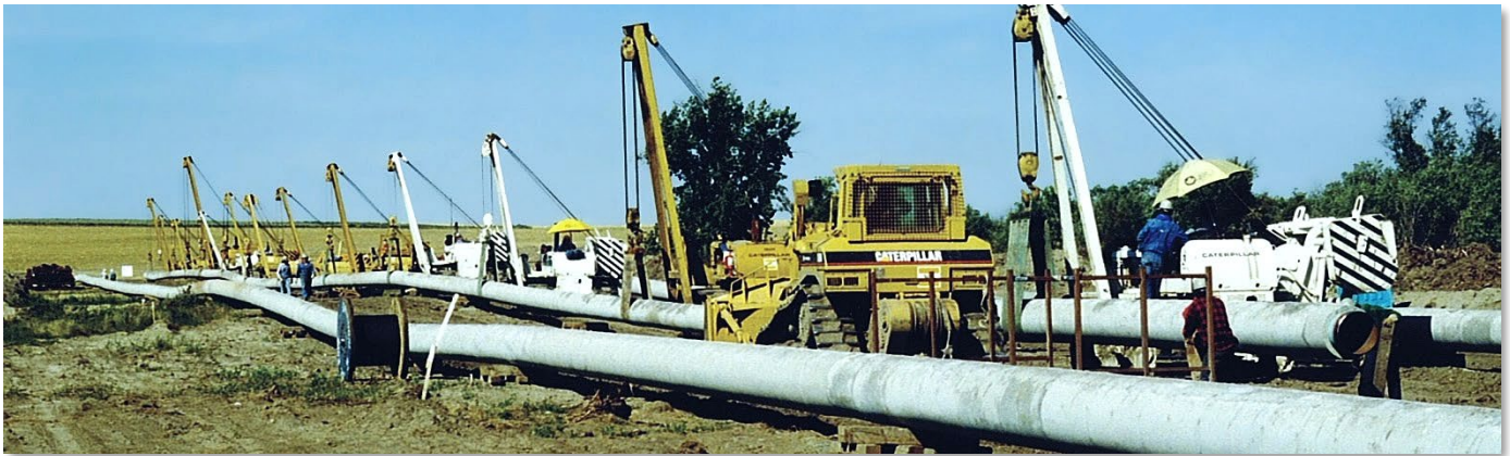
A below surface pipeline system is expected to comprise a process water pipeline to the processing plant at the mine and a return slurry pipeline conveying iron concentrate to the Cape Hardy Industrial Port Precinct (illustrative image).
