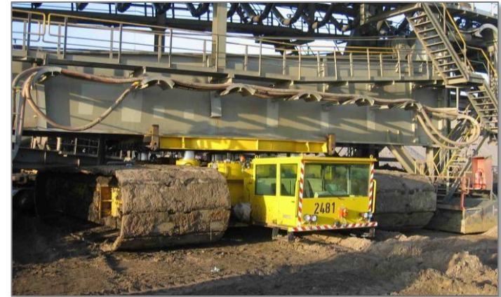
Top: Semi-mobile gyratory crusher station in Sweden, similar to capacity required at CEIP. Above: Transport crawler undertakes conveyor system reconfiguration
