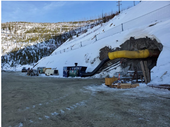
Portal Bench infrastructure supporting underground activities
