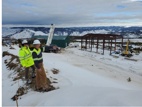
Surface facilities overview
