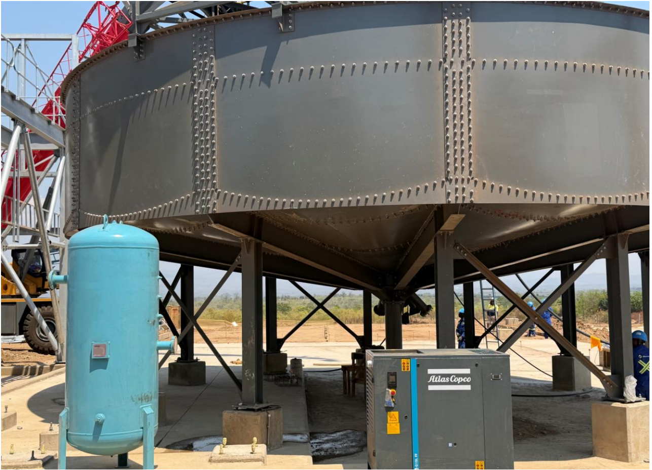
Picture 5. Thickener installed at process plant
