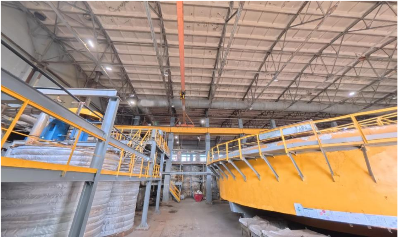
Picture 14. Existing processing infrastructure within the SARECO MREC Facility
