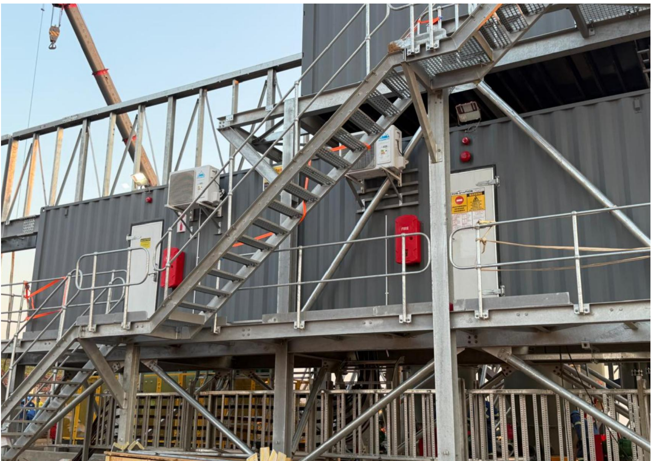
Picture 6. Motor control centres at process plant ahead of electrical commissioning
