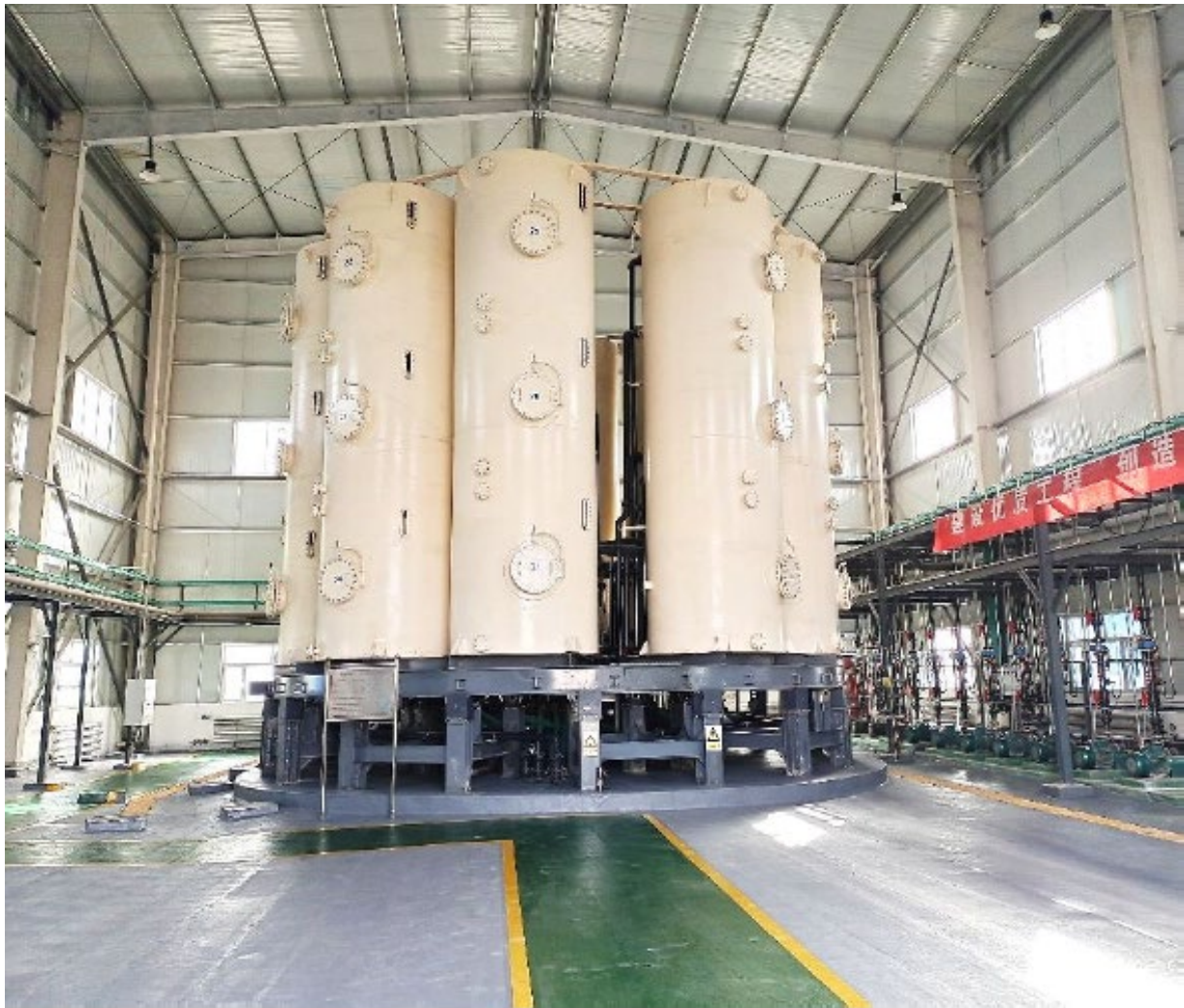
Figure 15: Lithium Adsorption Module of Lanshen Demonstration Plant, China
