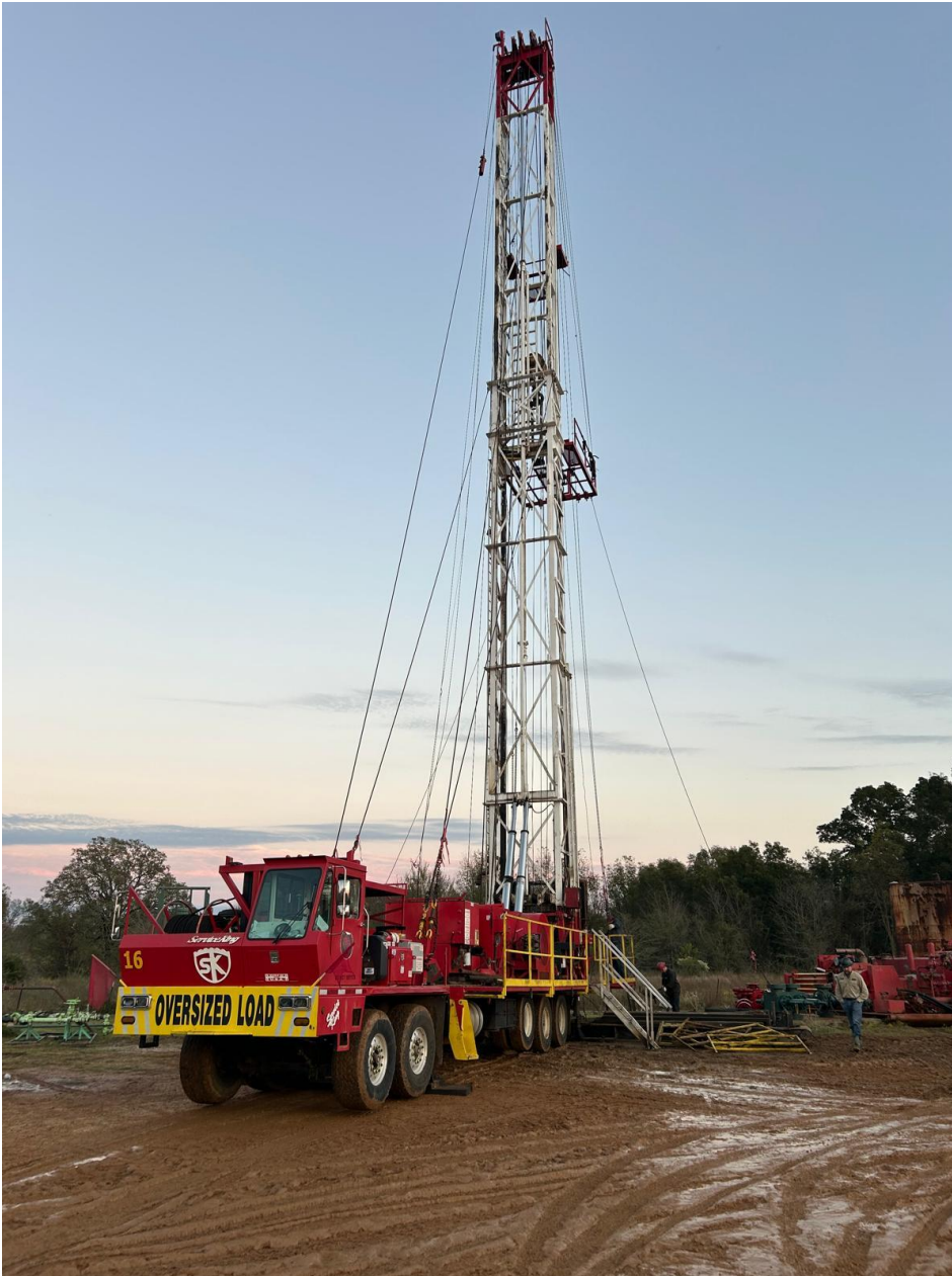
Figure 2. Rig on site at the first Pantera Smackover Lithium Brine re-entry test well in Lafayette County Arkansas
