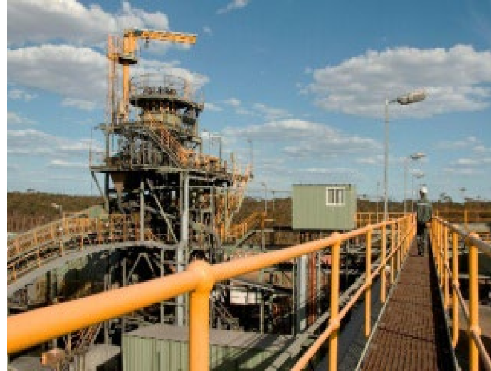
Lake Johnston processing plant
