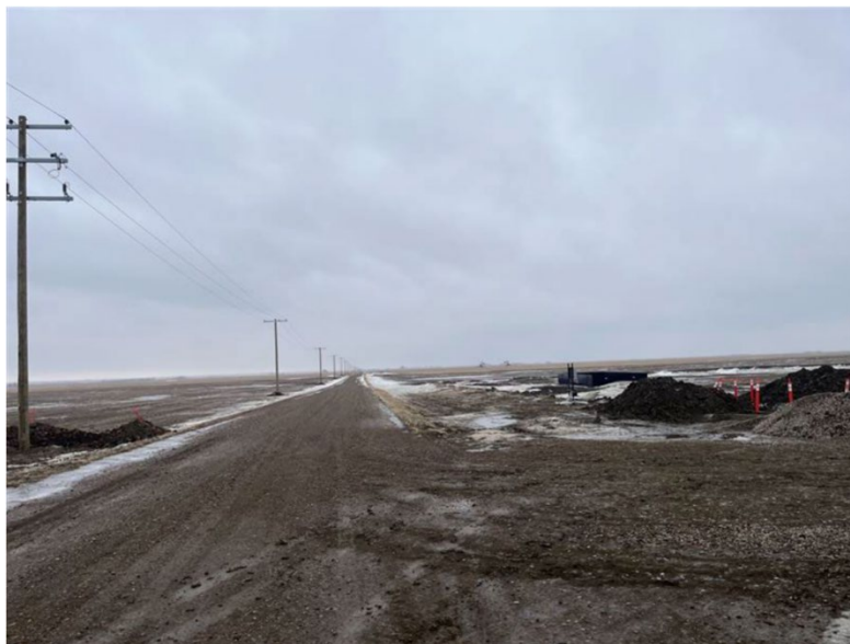
Figure 2: Power infrastructure installed at Pad #1
