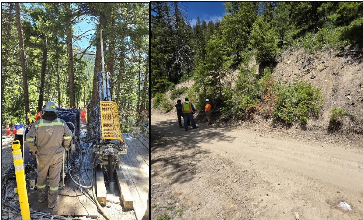
Figure 2: LEFT: Drilling Rig 03 (Left) at hole HH-GG26-004 on Ds10; RIGHT: Ds8 after drilling is completed. Three holes were drilled on Ds8 (HH-GG26-010, (HH-GG26-011, and (HH-GG26-012). Taking advance of the placing the drill sites on and very close to the access tracks, the rehabilitation is such that there is no visible trace of the drill collars.
