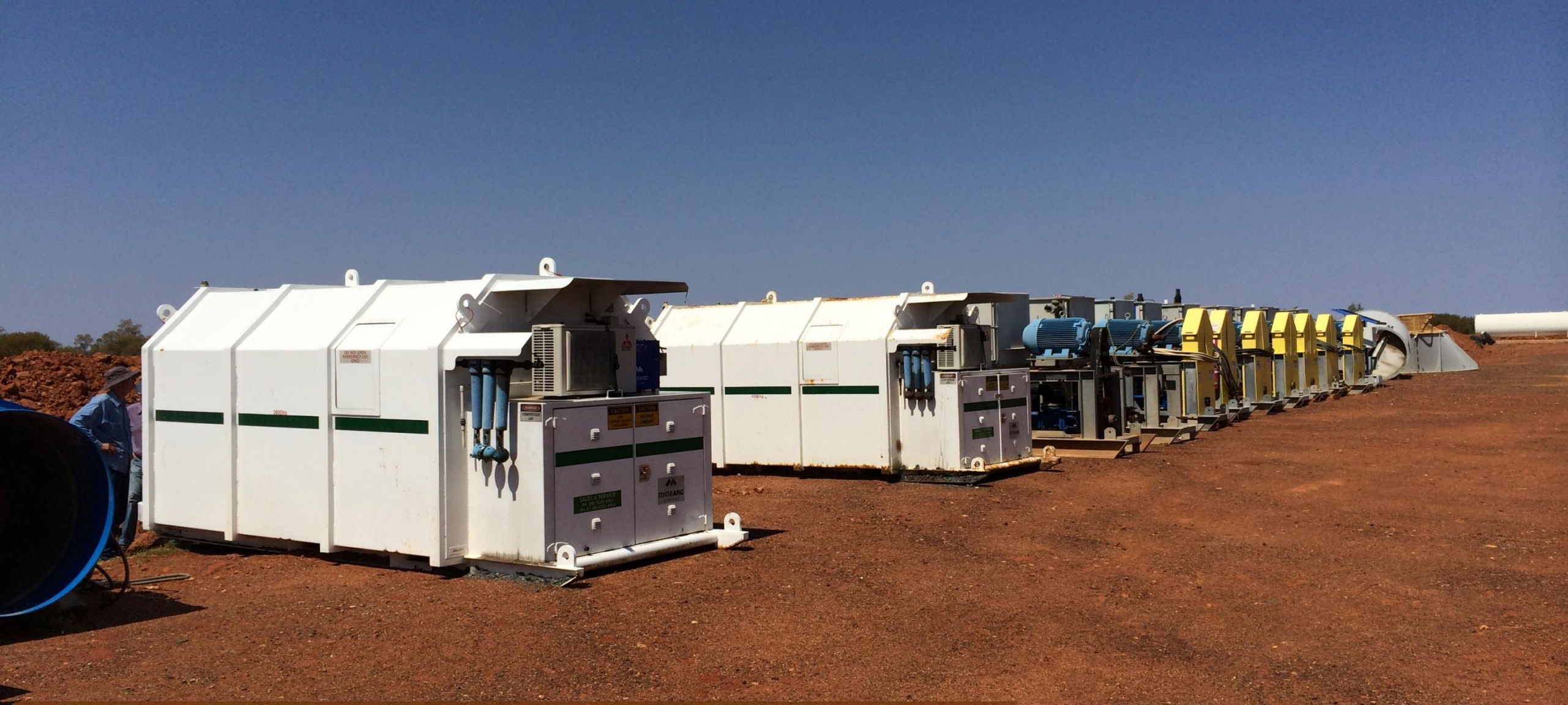
Sinclair Nickel Project – Underground Refuge Chambers and Mine Ventilation equipment
