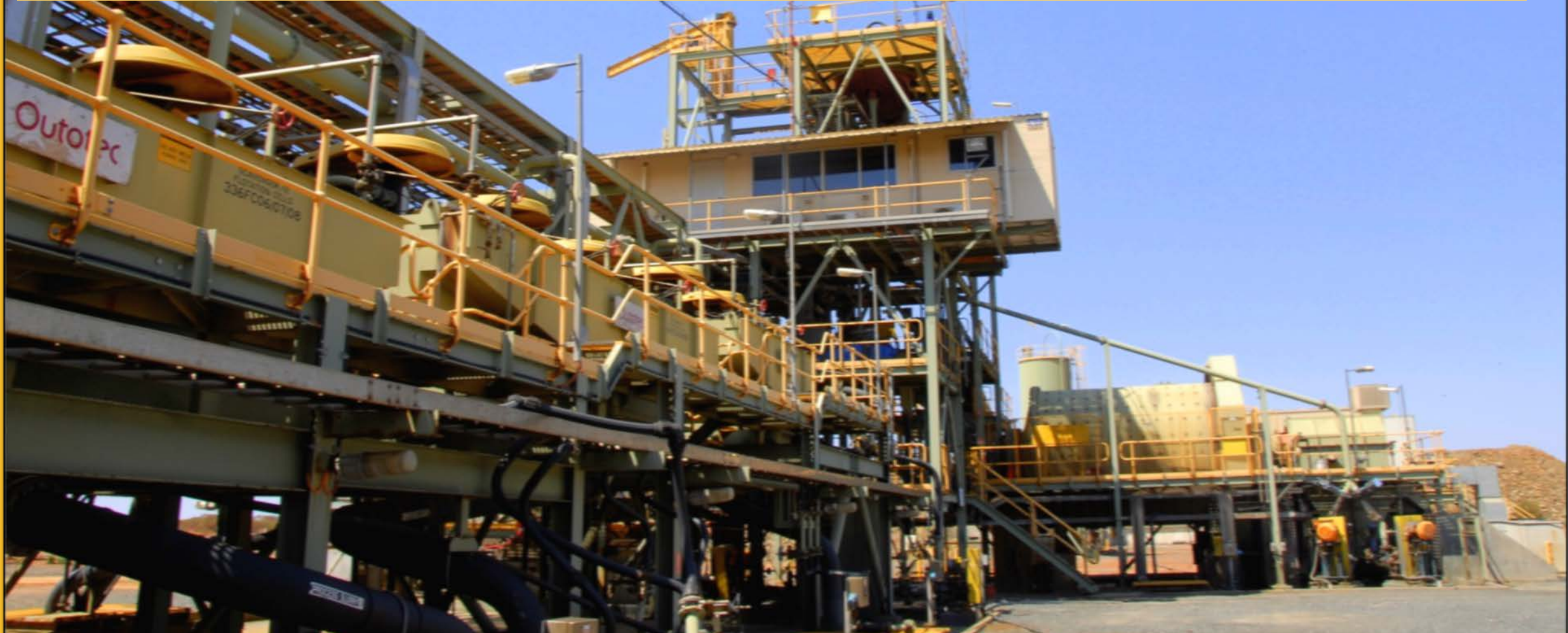
Sinclair Nickel Project – Flotation Cells and Mill Control Room
