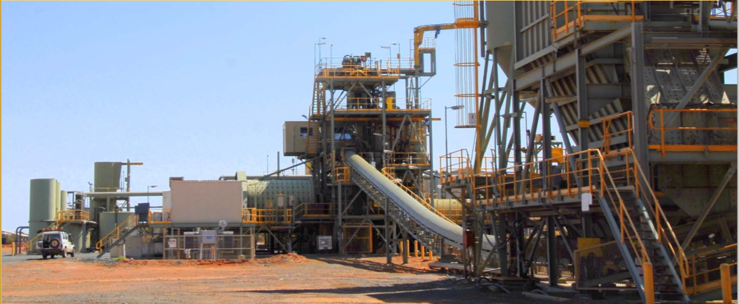
Sinclair Nickel Project – 300ktpa Crushing and Grinding Circuit
