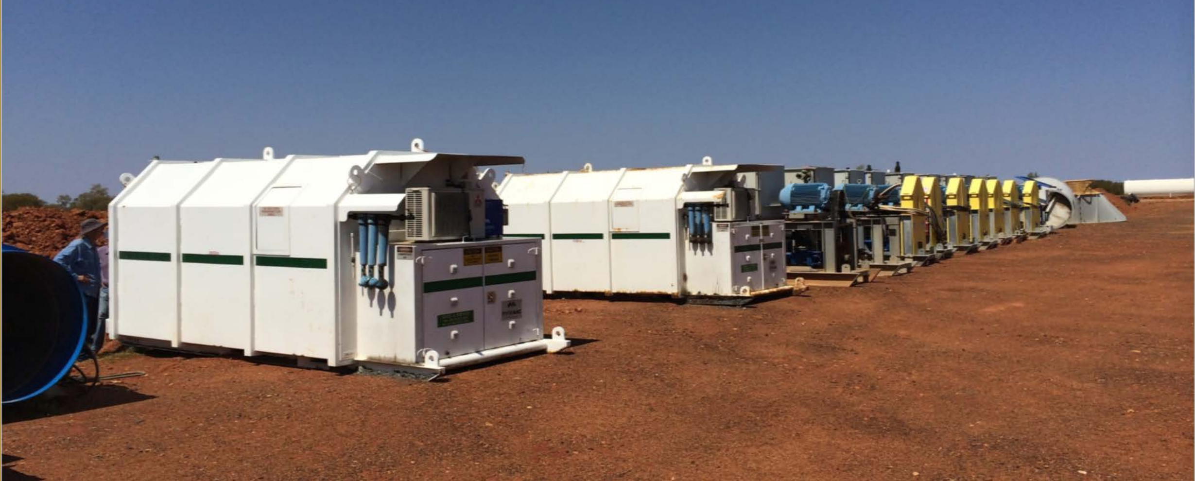
Sinclair Nickel Project – Underground Refuge Chambers and Mine Ventilation equipment
