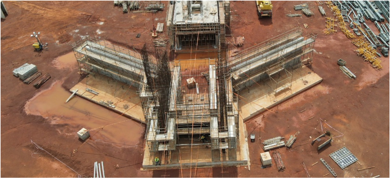
Figure 4: Crusher and reclaim chamber
