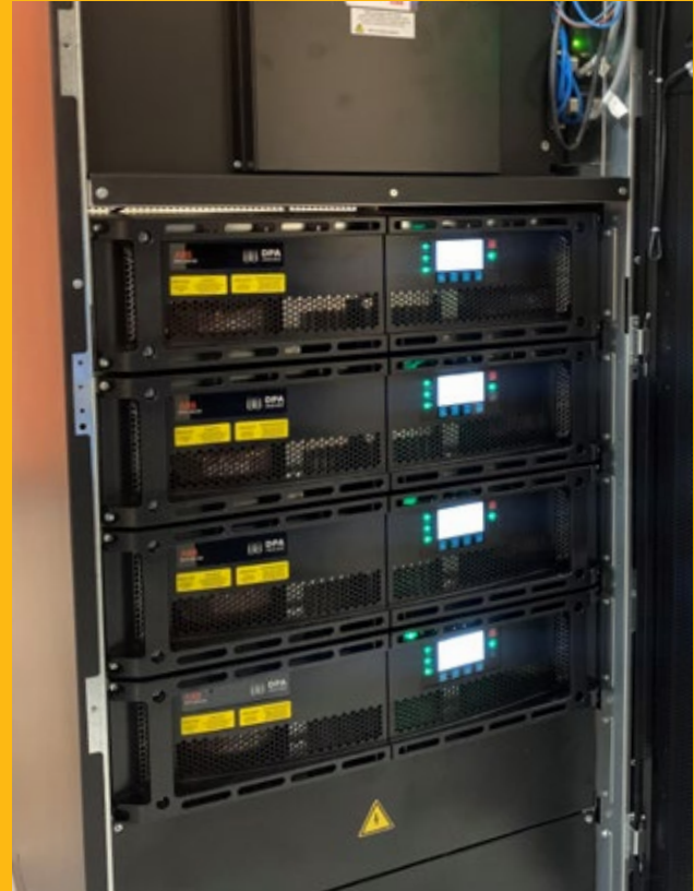
Data centre at Glebe, NSW.
