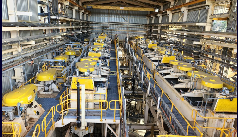
Outotec Flotation cells within Flotation Building
