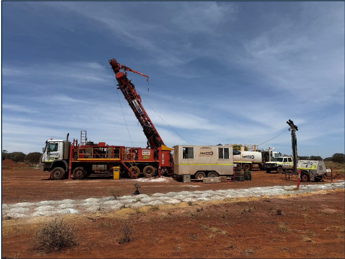
Figure 3: Diamond drill rig set-up and drilling on 24IWBR0039, completing a diamond tail on the Siona discovery hole.
