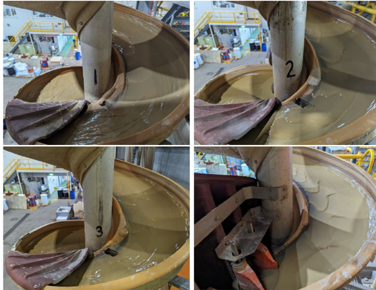
Figure 6 - Wet Concentrator plant, Rougher Spirals
