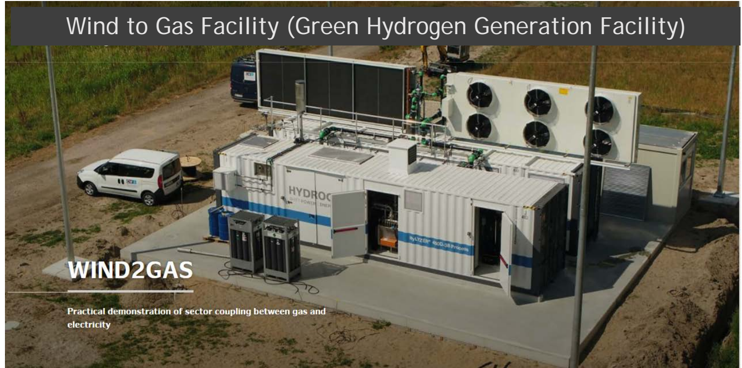
Brunsbüttel, Hamburg, 2.4 MW electrolyser facility
