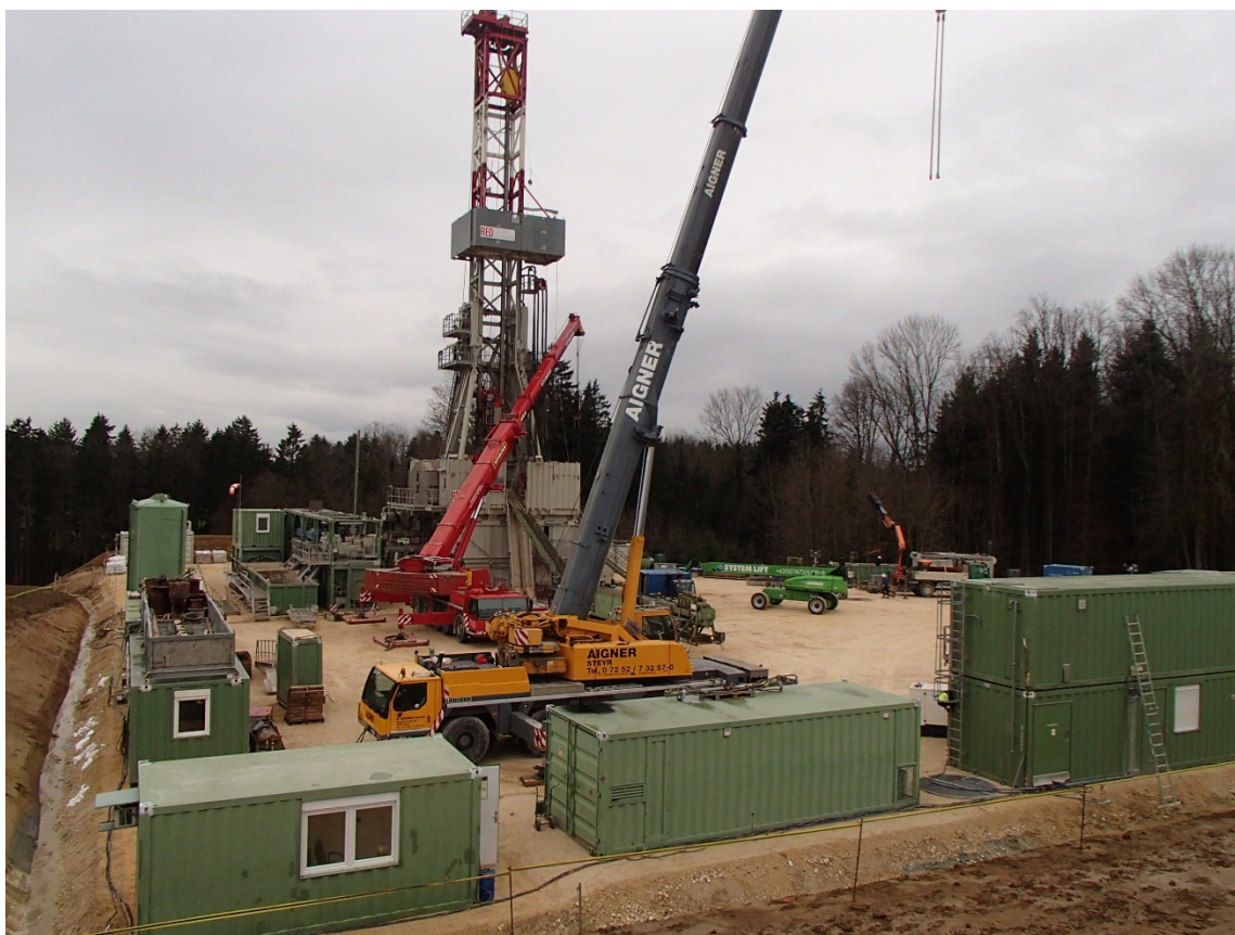
Figure 1: Rig up of RED E-220 rig in preparation for Anshof-3 well spud
