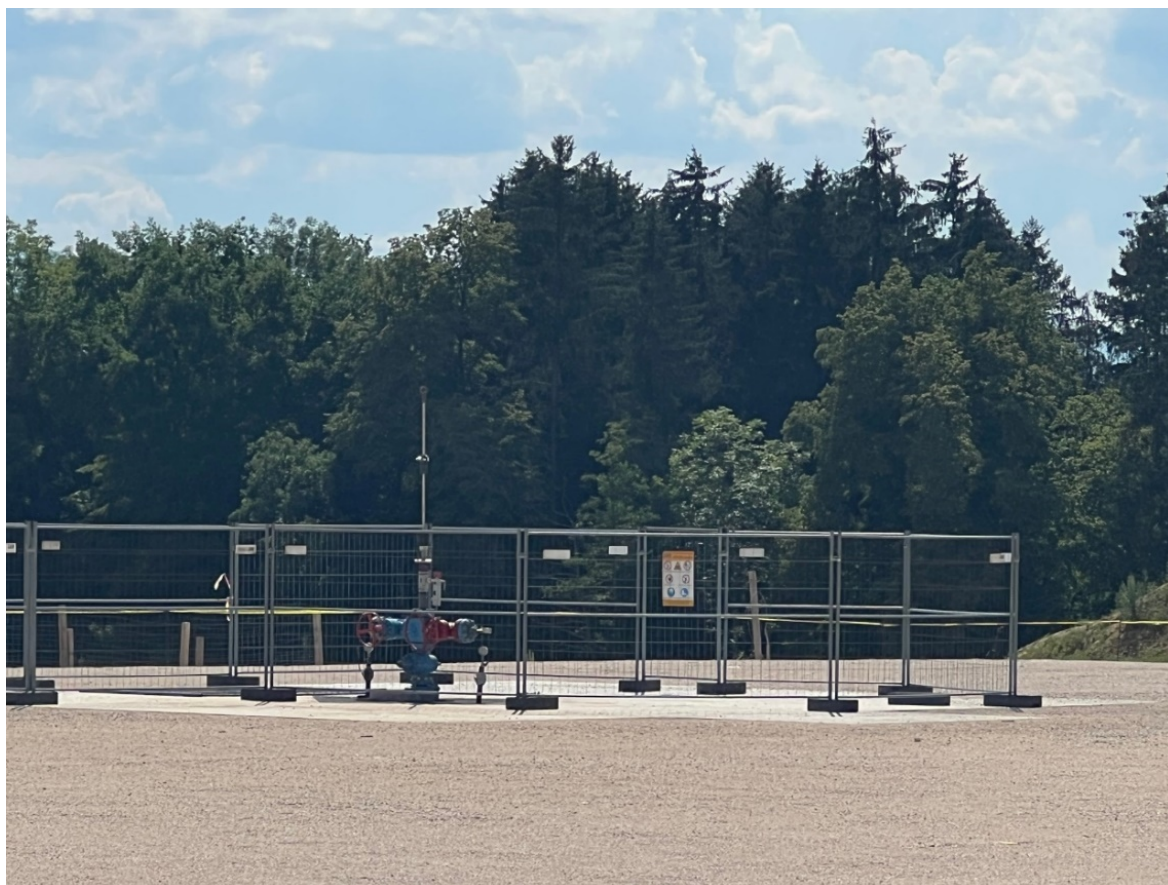
The Anshof- 3 well location showing the installed well head operationally ready for production. Source ADX
