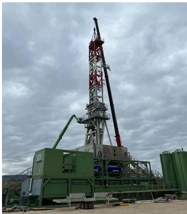
Figure 1: Rig up of RED E-202 rig in preparation for Anshof-2 well spud
