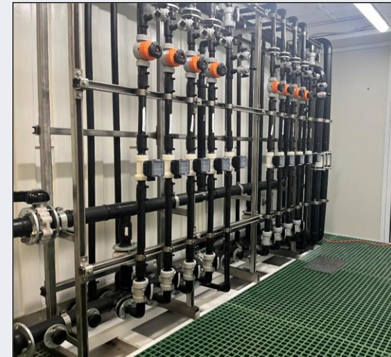
Wellhouse Module (pipe room)
