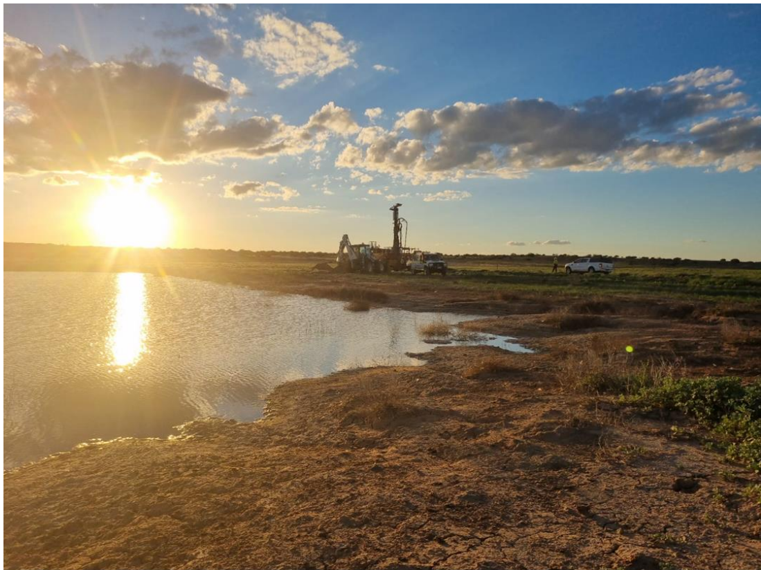
Figure 5: Photo of Alligator's contractor (Wallis Drilling) drill rig at Big Lake Project.
