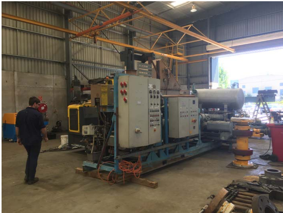
Image 2: Paddle dryer pilot skid at Bossong Engineering in Perth for maintenance and modifications
